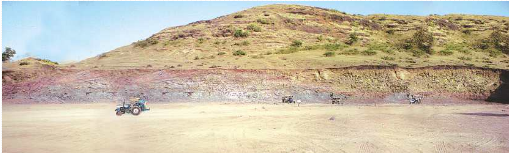
Site : Beru India Ltd. MIDC Talegaon, Pune. Client : Kakkad Constructions, Pune Work Nature : Land development Contract Value : 2 CR For Ref. : Mr. Amrish Kakkad Mob No: +91 9823020700
