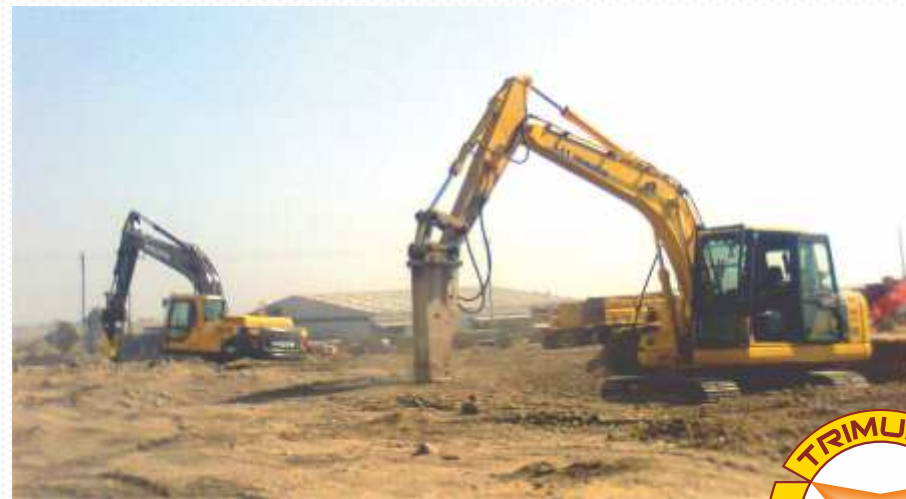
Site : Tenneco Automotives, MIDC Chakan, Pune Client : Reward Construction Pvt Ltd. Pune Work Nature : Earthwork Contract Value : 2.5 CR For Ref. : Mr. Ranjit Mohokar (Project Manager) Mob No: +91 8600101209
