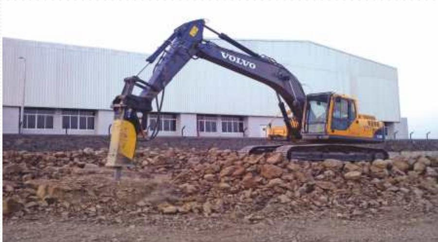
Site : Gebirit International, MIDC Chakan, Pune Client: Transtech Turnkey Projects, Pune Work Nature : Land Development & Road Work Contract Value : 2 CR For Ref. : Mr. Wankhede (Project Head) Mob No: +91 9861234963
