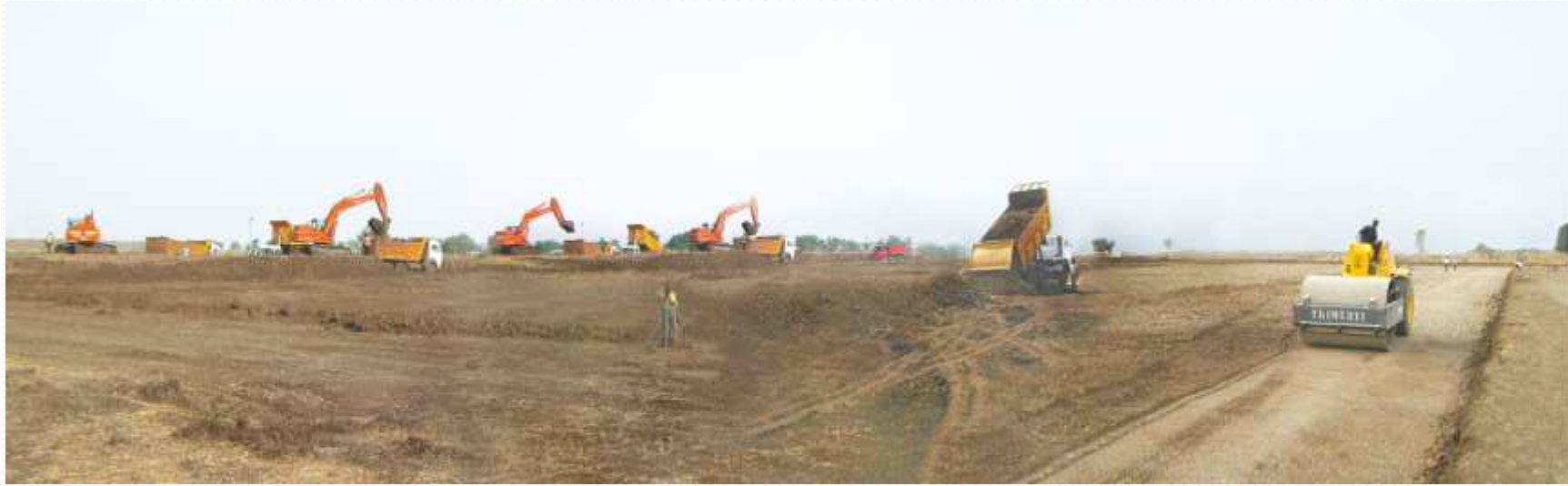
Site : Wheels India Limited, MIDC Deoli, Nagpur. Client : Reward Constructions Pvt. Ltd., Pune Work Nature : Land development work Contract Value : 3 CR For Ref. : Mr. Ranjit Mohokar (Project Manager) Mob No: +91 8600101209
