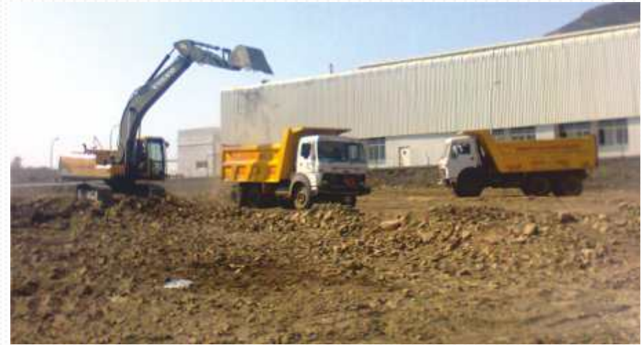
Site : Mahindra & Mahindra, MIDC Chakan, Pune Client: Reliable Constrotech Enterprises Pvt Ltd. Mumbai Work Nature : Earthwork. Contract Value : 2 CR For Ref. :Mr. Pravin Sarode (Project Manager) Mob No: +91 9819001449
