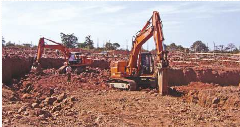
Site : Auditorium, Sankwal, GOA. Client : Klasic Construction, Mumbai Work Nature: Land development Contract Value : 1 CR For Ref. : Mr. Motwani (Director) Mob No: +91 9833831346
